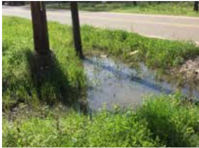
Existing drainage conditions on Lake Drive Photo Credit: UNO Team
