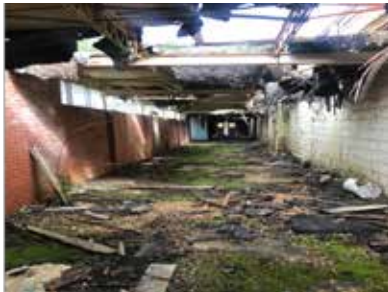
Current condition of Campti High School site, Campti, LA Source: UNO Team
