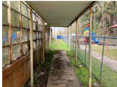
Current condition of Campti High School site, Campti, LA Source: UNO Team
