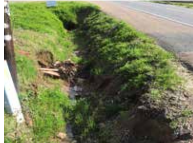
Existing drainage conditions U.S. Route 71 Photo Credit: UNO Team
