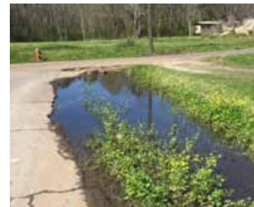
Flooded right-of-way on Lake Dr. Photo Credit: UNO Team
