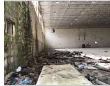
Current condition of Campti High School site, Campti, LA Source: UNO Team
