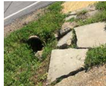
Collapsed sidewalk on Mill Street Photo Credit: UNO Team
